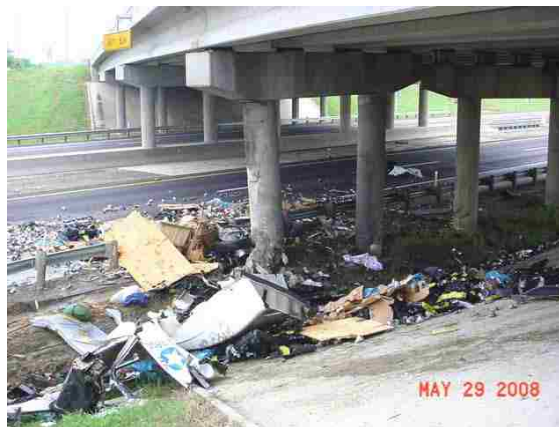
Figure 2.7. Truck-tractor-trailer accident–FM 1401 Bridge, Texas, 2008 (Buth et al. 2010)
