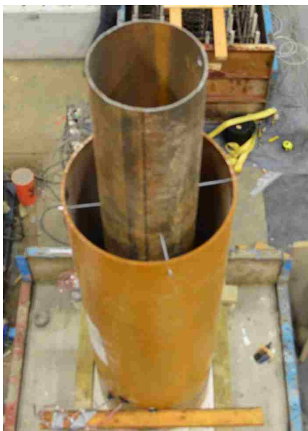
Figure B.8. Install the formwork of the RC-column and the FRP tube for the HC-FCS column
