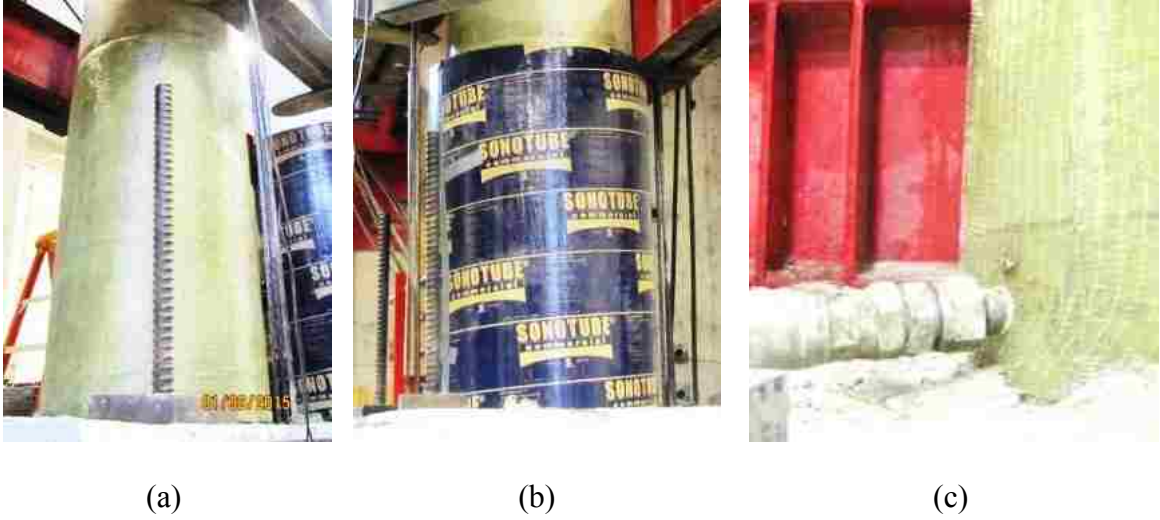
Fig. 2. Rapid repair of the C1 column: (a) wrapped GFRP, (b) heat chamber, and (c) grout injection
